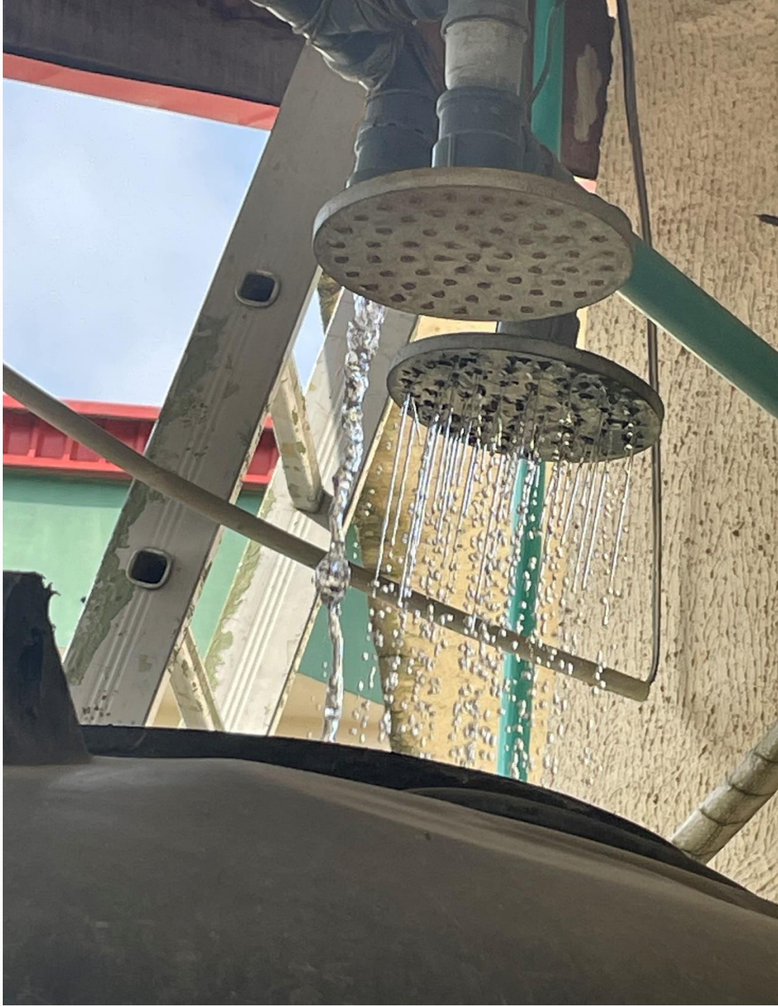
Figure 2.5 Showering of water for aeration. (MTU Factory)
