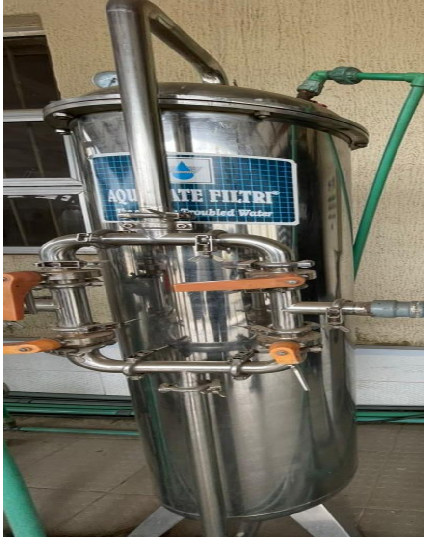
Figure 2.8 Resin filter (MTU Factory)
