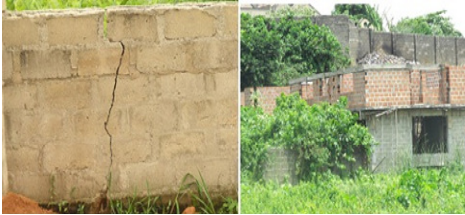
Figure 1. Samples of affected building structure from the area.
