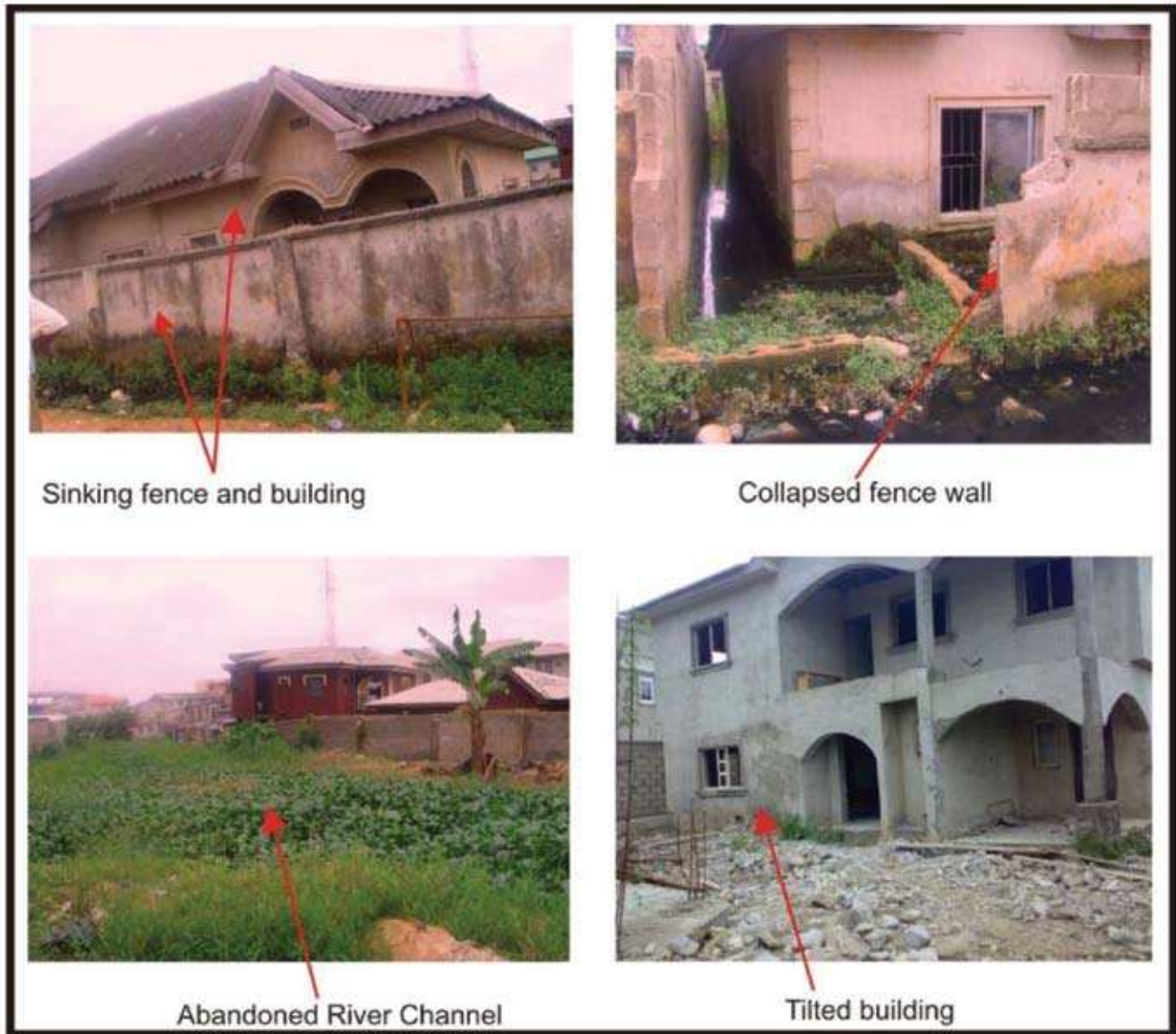
FIGURE 4. Different Degrees of Structural Instability Observed on Buildings in the Area
